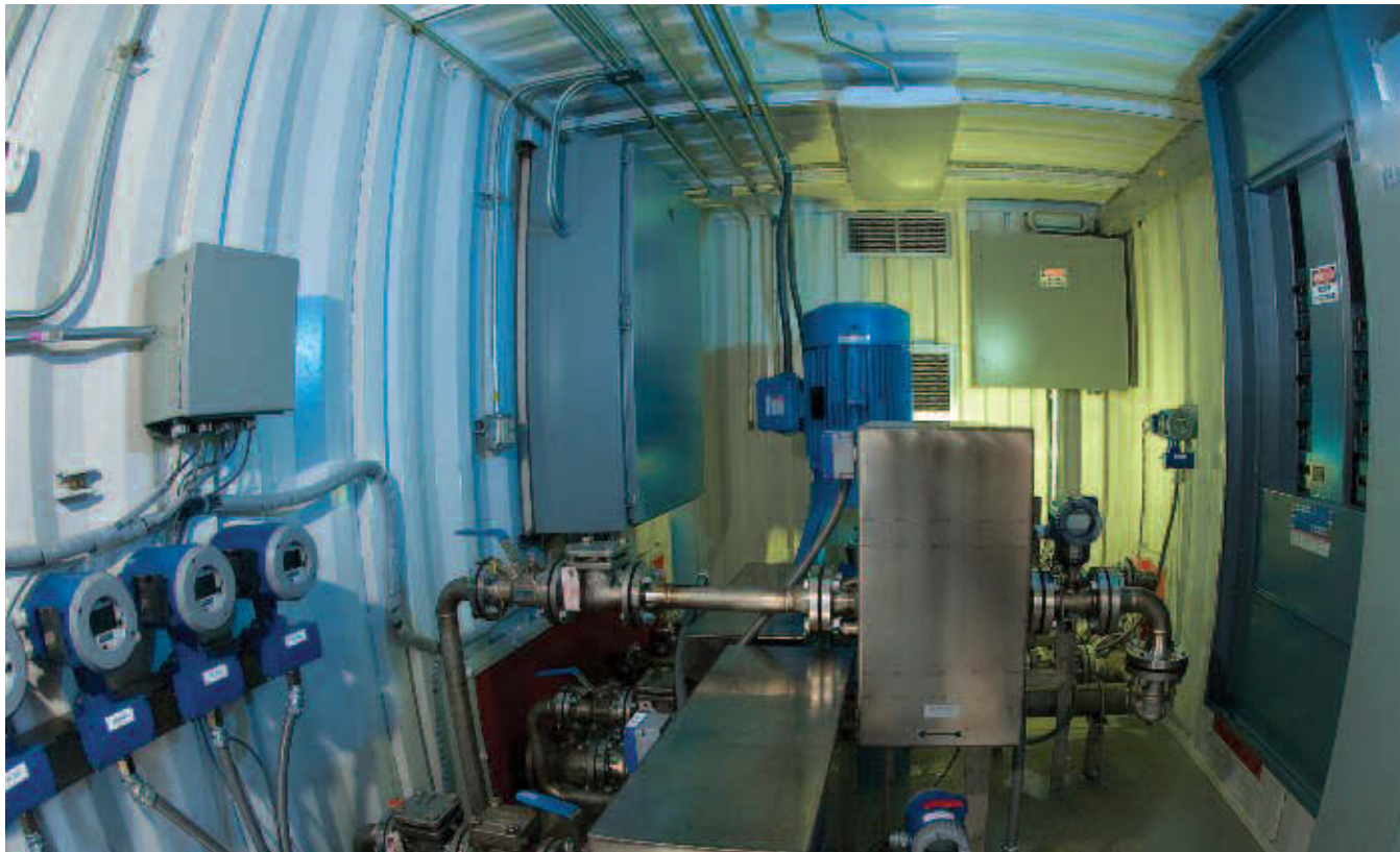
DMT is a fast, effective, and environmentally safe innovation for removing steam generator secondary side deposits.
