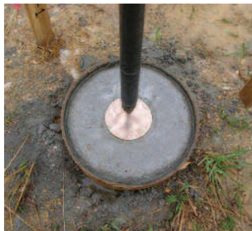
Preparation for Calvert Cliffs unit 3 continues, with installation of survey monuments at strategic locations.
