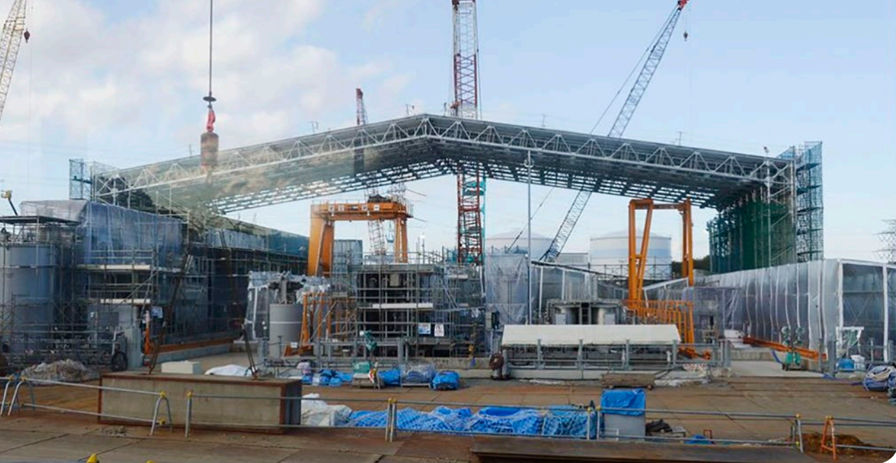
Construction of the ALPS processing facility on the Fukushima Daiichi site in 2013. Photo: TEPCO
