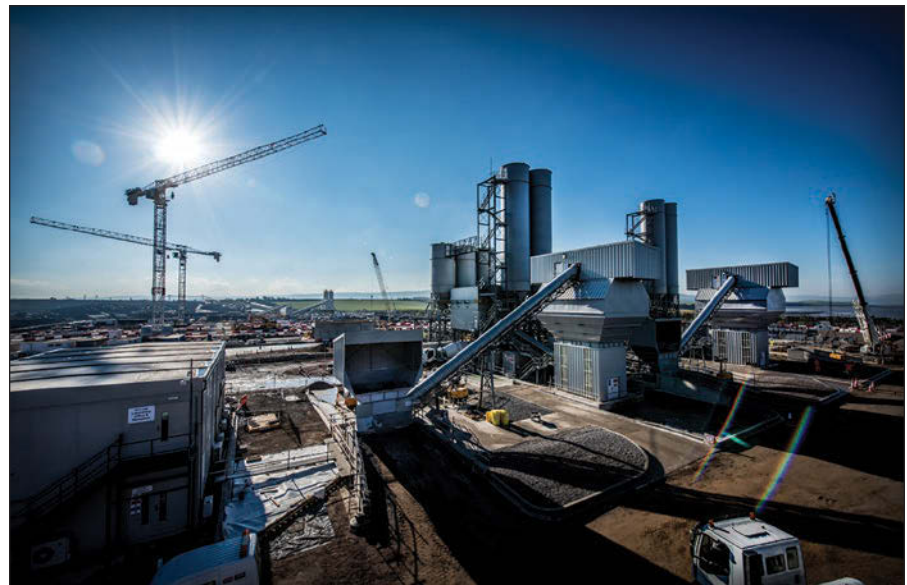
The photo above, taken in January 2017, shows the concrete laboratory (at left) and two concrete batching plants at the construction site.
