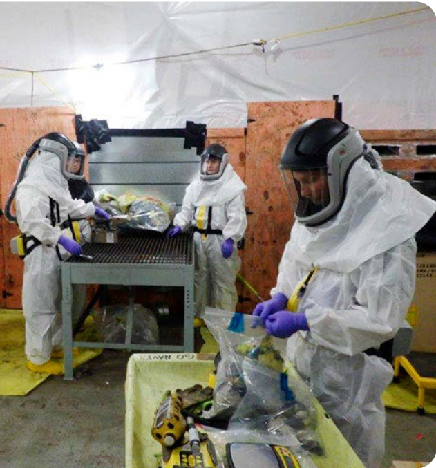
Workers sort through legacy items inside the Alpha-4 building to prepare for the facility's deactivation at Oak Ridge's Y-12 National Security Complex. (Photo: DOE)
