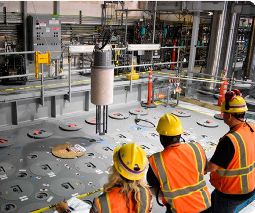
Workers install one of 18 startup heaters into Melter 1 of Hanford's Low-Activity Waste Facility. (Photo: Bechtel National)
