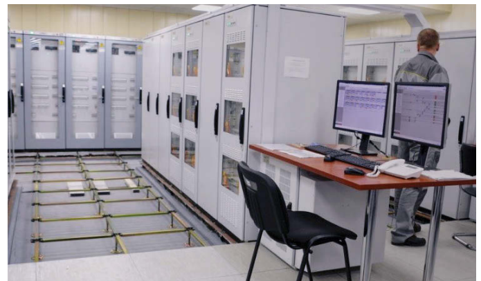
Digital safety systems require fewer equipment racks, reducing the total data center footprint.
