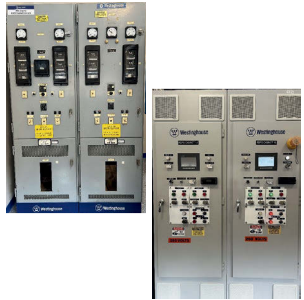
Original MG Cabinet (left) vs. Next Generation Replacement MG Cabinet (right)
