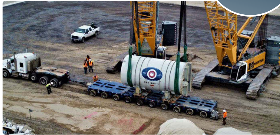
The Savannah 's reactor pressure vessel arrives at a licensed low-level radioactive waste disposal facility in Clive, Utah. (Photo: EnergySolutions)
