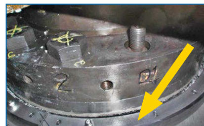
Reactor recirculating pump protected by AEGIS® RPPR.
