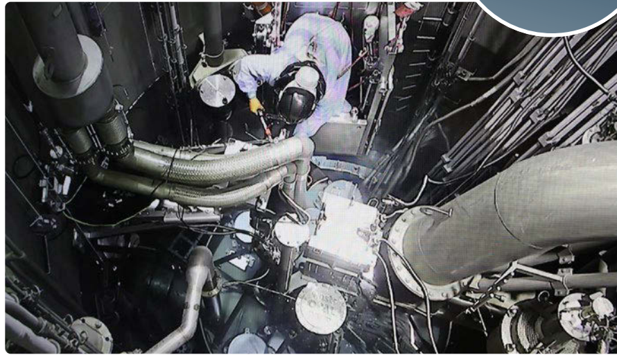
A technician works inside OPAL's reactor vessel during the maintenance and upgrade project. (Photo: ANSTO)
